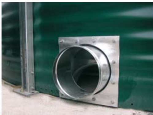
Photo: silo connection nozzle
