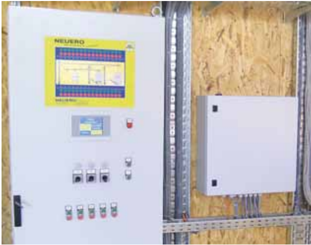
Touch panel in a NEUERO switching cabinet
