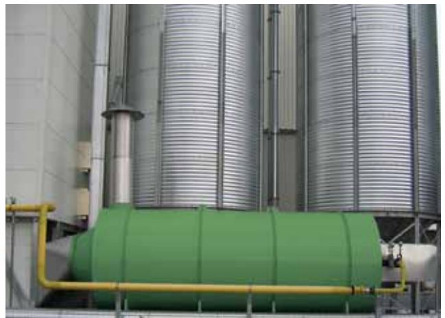
Indirect hot air generation with an oil burner
